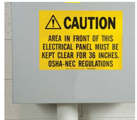
Hazard warning signs
