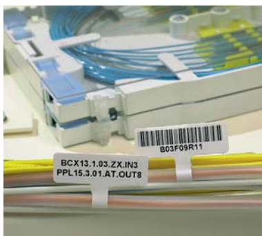
Fibre Optic Cable Markers
